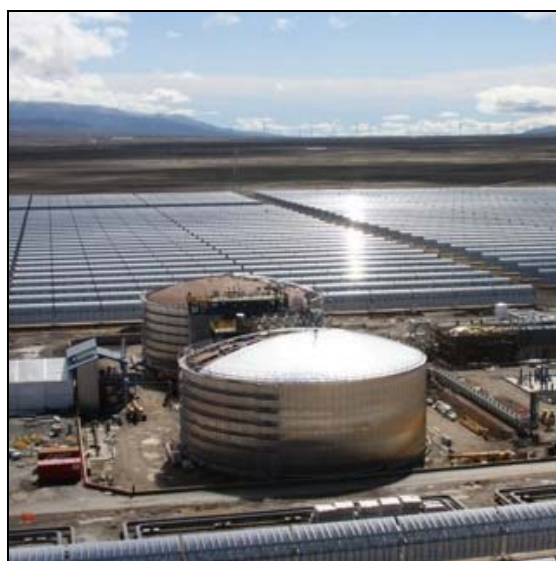
Figure 35. Two-Tank TES System at a 50 MW Solar Power Plant in Spain
